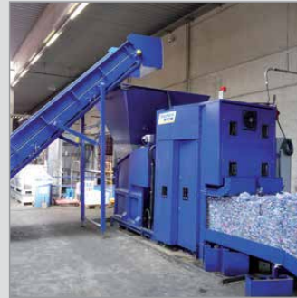
Loading by means of a conveyor belt
